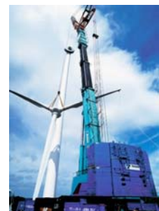
All terrain crane lifting blades for assembly of an offshore wind turbine
