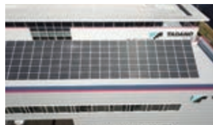
Solar panels installed at Advanced Technology Research Center
